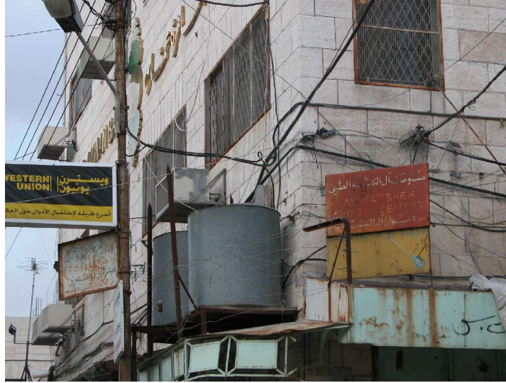
Figure 2-15: External electrical wires on the walls of Al-Ahli Bank in Al-Shalalah District. Source: The author, 19 th of September, 2004
